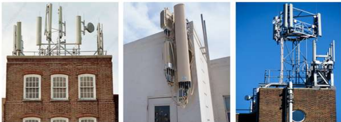
Figure 2: Building mounted base station (left), rooftop base station (middle), and mast installed on building (right)
